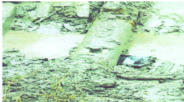
SPILL POINT AFTER EXCAVATION
